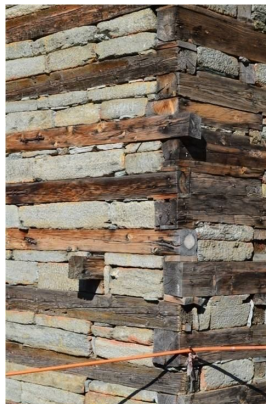
Figure 8: Courses of stone and wood placed to form the wall- Kath kuni Construction (Source: Author)
